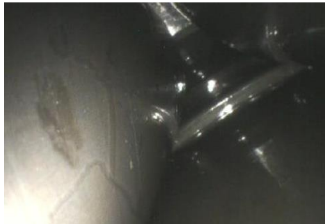
Figure 13 - Boroscopy results for the generator-side HSS bearing (HS-S-GS)
