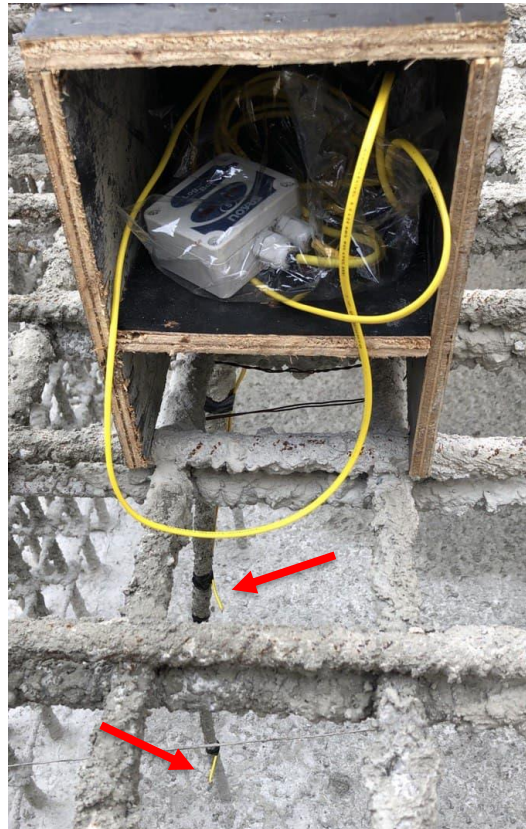
Figure 13 – Thermocouples installed in the reinforcement before the pouring of a foundation structure
